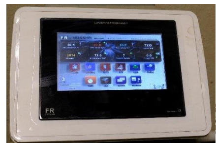
Figure 3: Temperature, humidity and gas monitoring control panel of the barn
